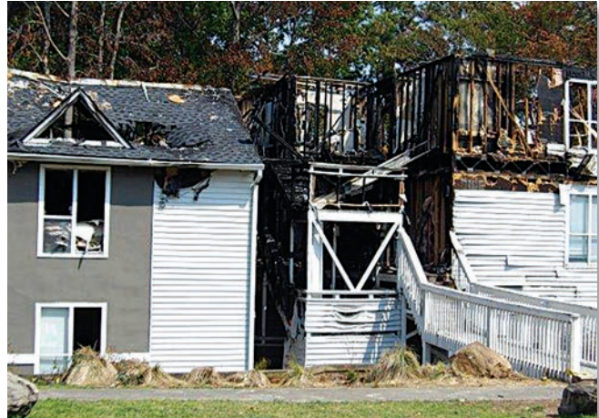
Front view of fire damage to building
