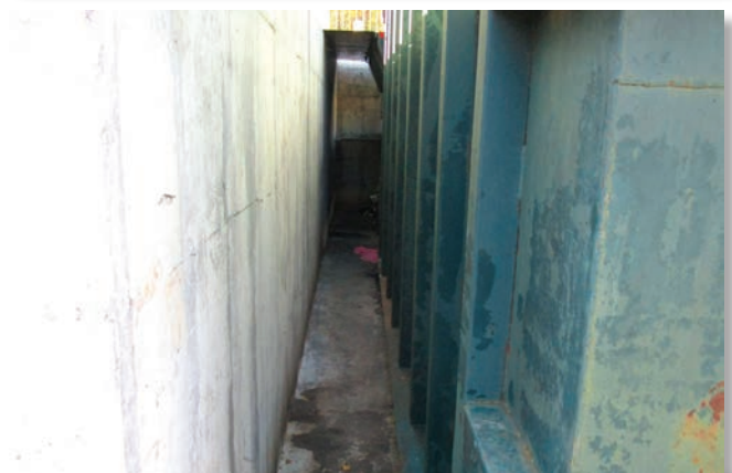
Area between the retention wall and household/garbage waste container where employee 1 was pinned.
