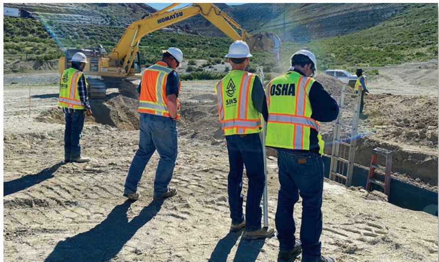
Members of the WYOSHA Compliance Assistance Program conduct a compliance inspection at a trenching worksite.
