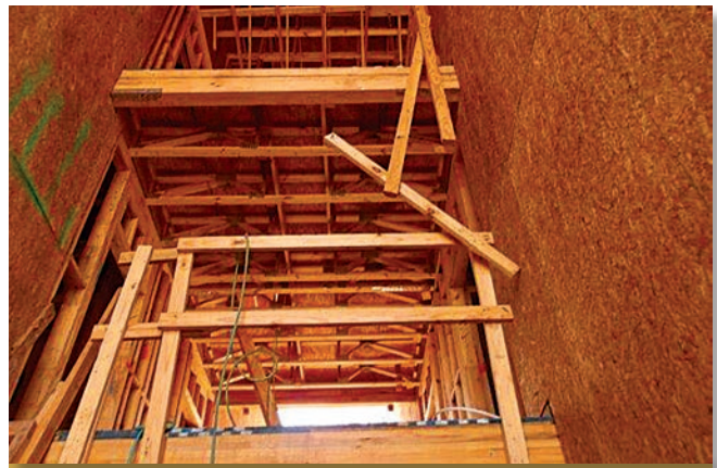
Close up photo of elevated area depicting the failed guardrails.
