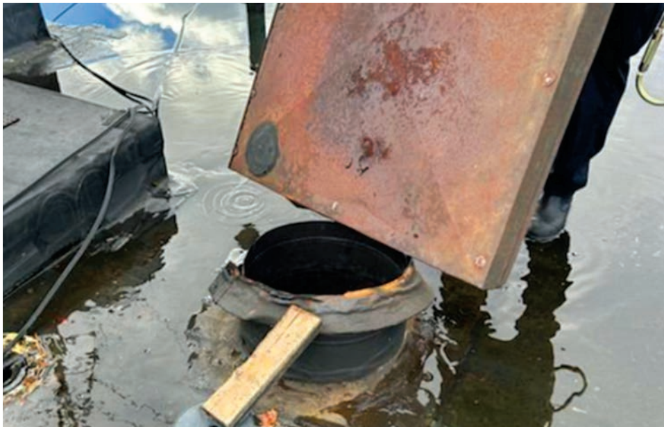
Photo of the steel plate that covered the exhaust vent stack for the third-floor boiler system.
