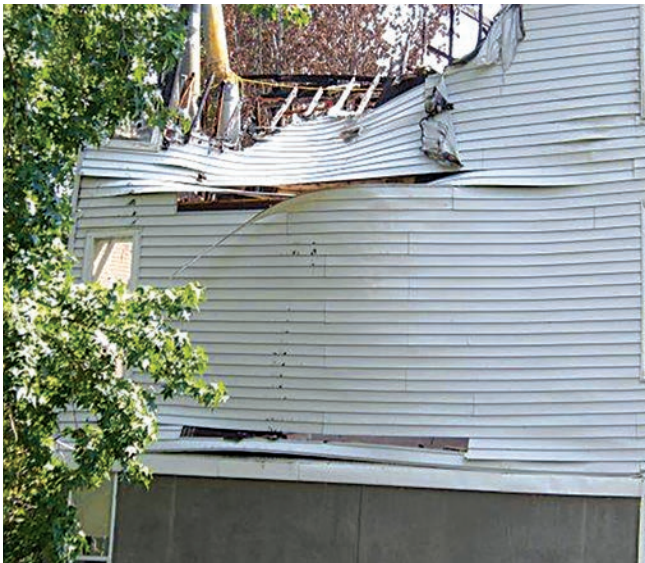
Back view of collapsed building due to fire damage
