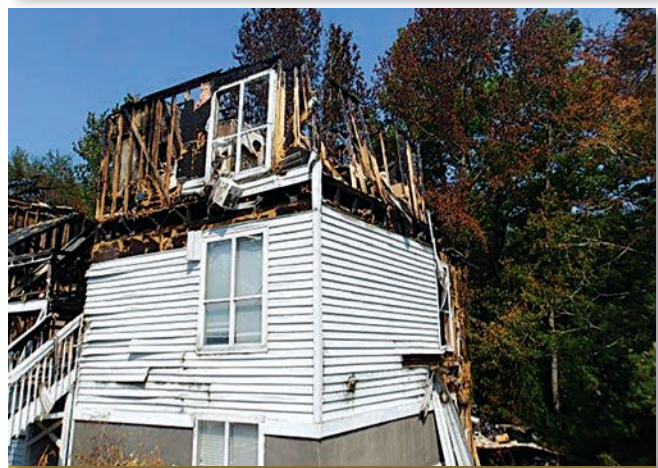
View of fire damage on side of building
