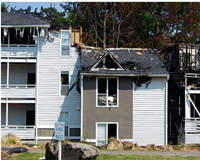
Additional front view of fire damage to building
