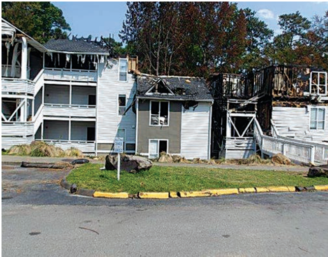
Front view of fire damage to building
