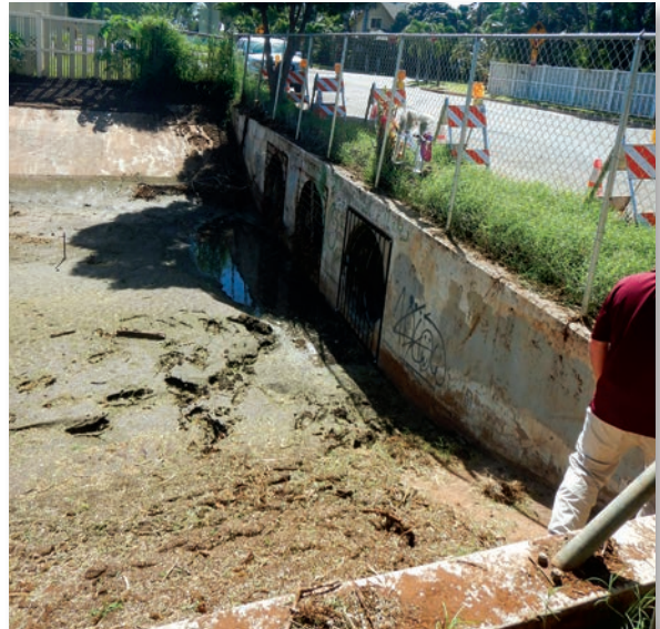
The submerged storm drainpipe is pictured following the death of a firefighter pulled into a sewer channel drainpipe.
