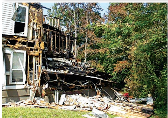
Side view of collapsed building due to fire damage
