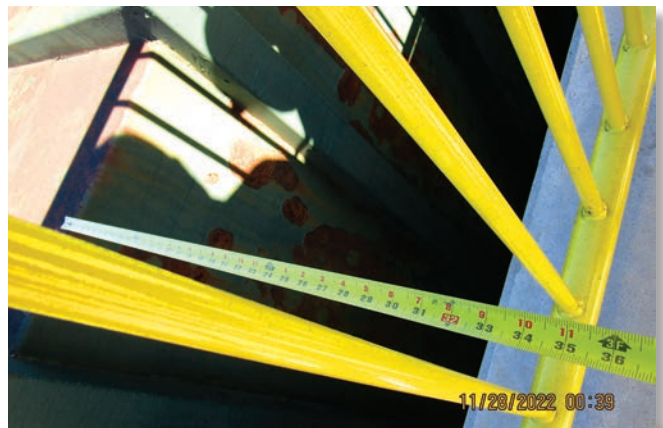
The area between the retention wall and the household/garbage waste container was approximately 33 inches.
