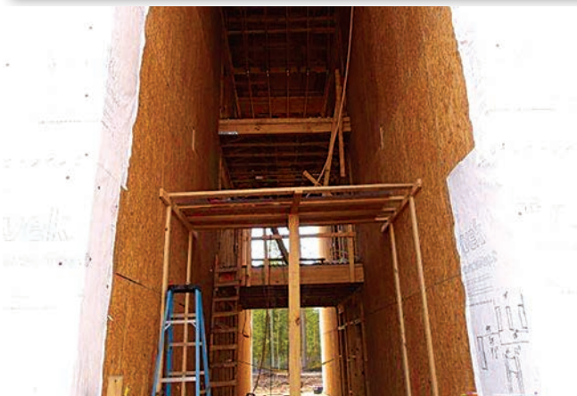
Third floor accident scene
