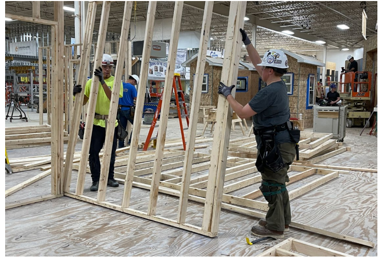
Jesus Sandoval and Carla Marsland hold framing at the Carpenters Training Institute.
