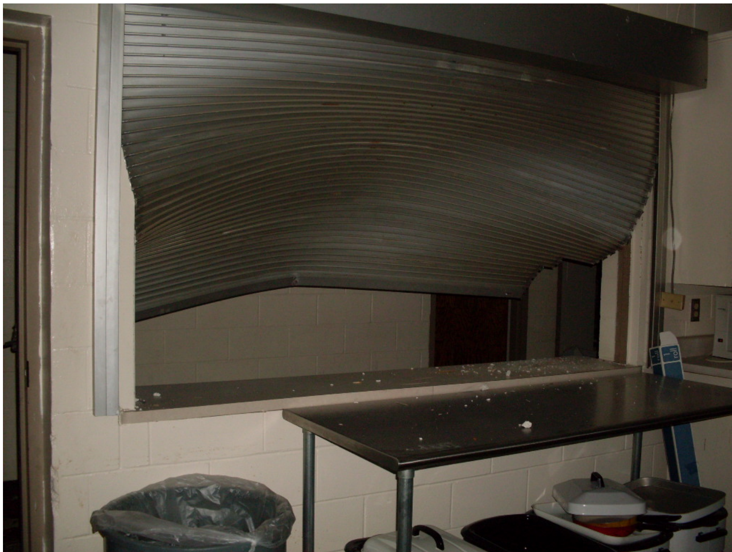
A photo of the damaged roll-up doors for the kitchen.
