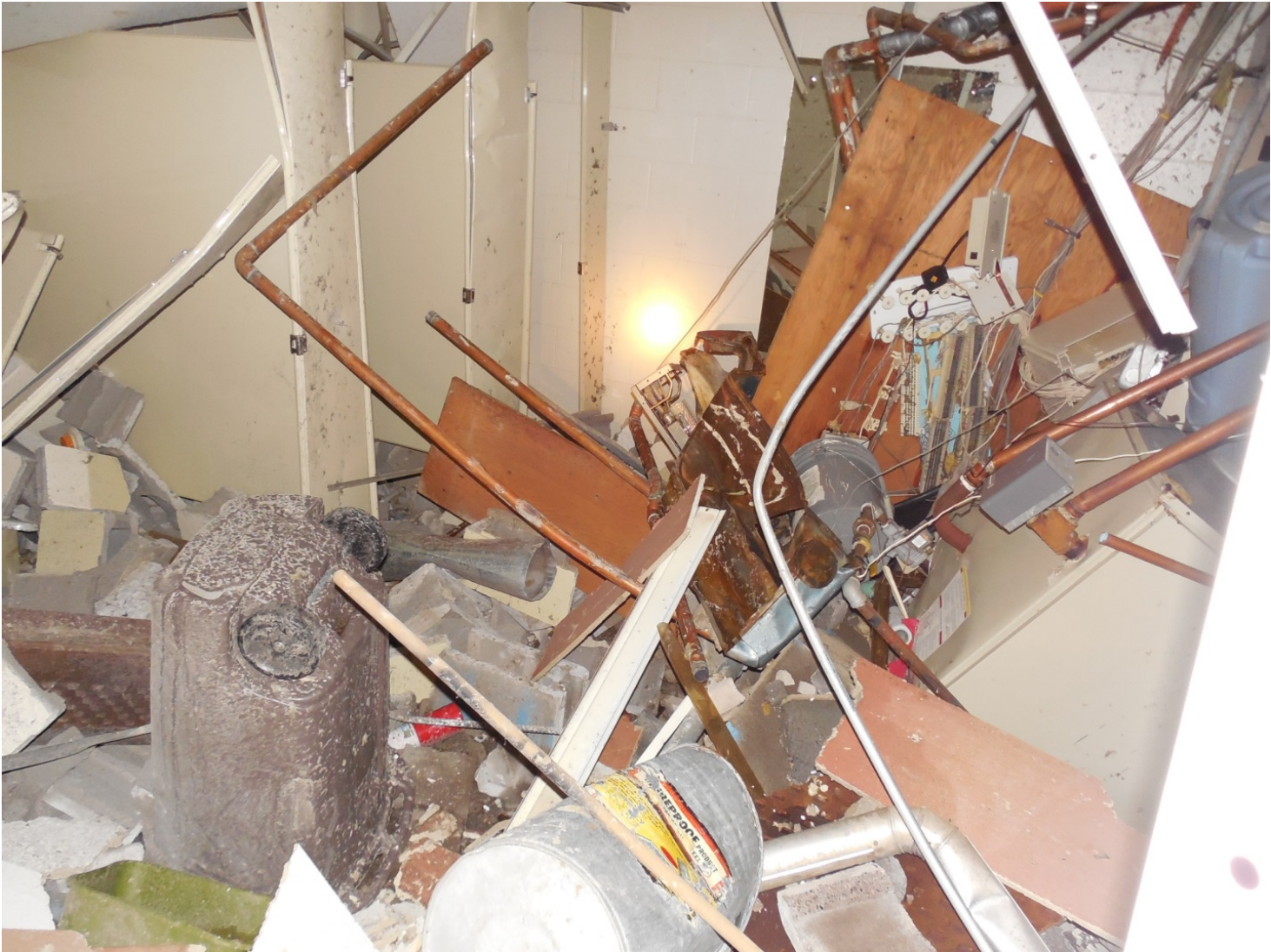
This image looks at the damage in bathroom from hallway near boiler room entrance. Notice the destruction of the bathroom stalls. These stalls were located 18 feet away from the boiler and behind a six-inch-thick concrete block wall.
