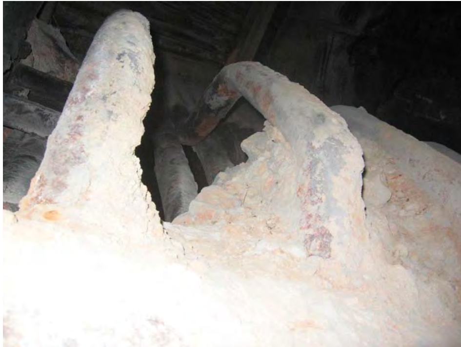
48. West side dead air space before ash is completely removed Note impacted ash between tubes above header (buried)
