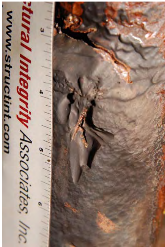
41. Close-up of Tube 9 middle leak
