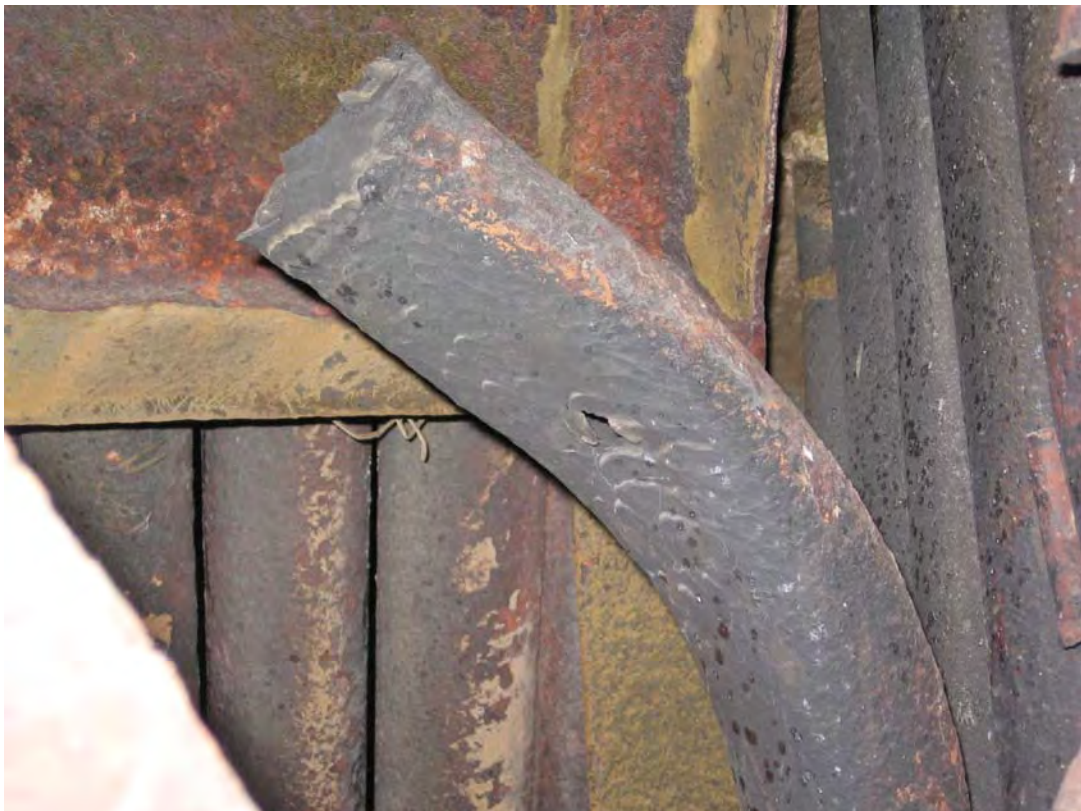
33. Tube 10 showing damage from steam / water impingement
