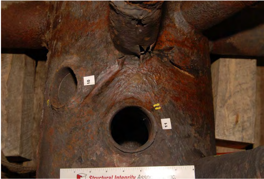
17. Overview of header at failure area
