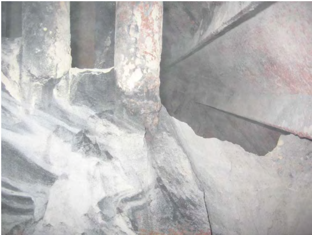
43. West side dead air space before ash is completely removed Tubes encased in ash going to lower header
