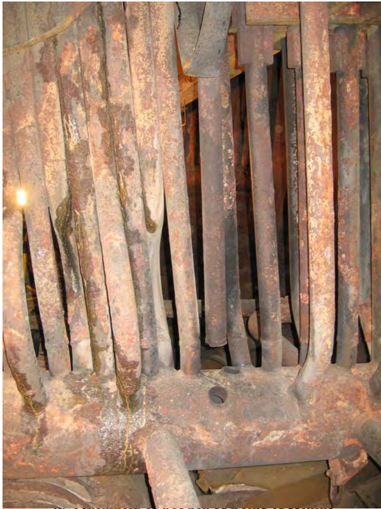
28. Overview of header at point of failure
