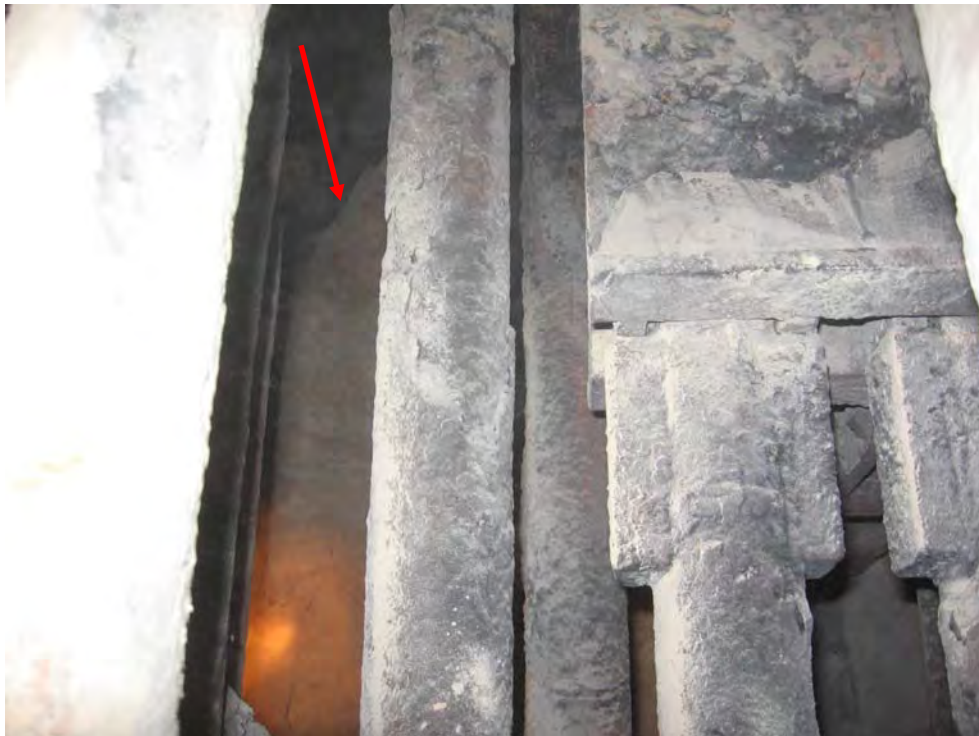
45. West side dead air space before ash is completely removed Note level of ash behind tubes.
