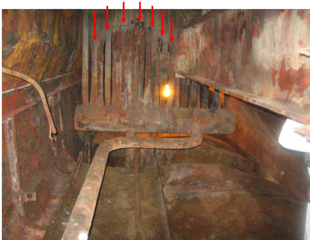
49. West side dead air space after ash is removed. Prior level of ash is evident on division wall header
