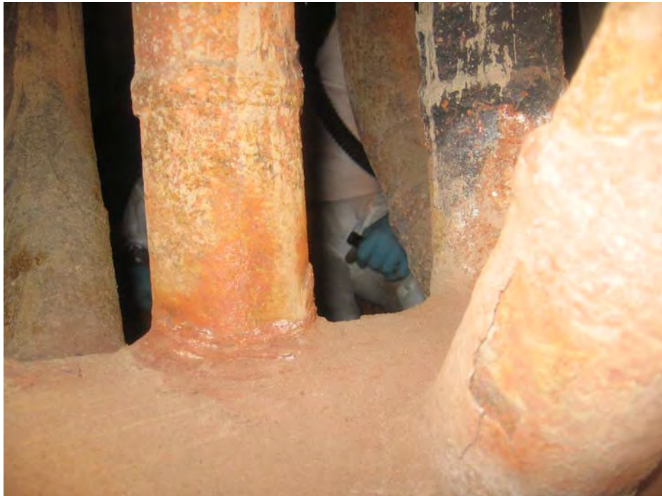
51. West side dead air space header after ash is initially vacuumed out
