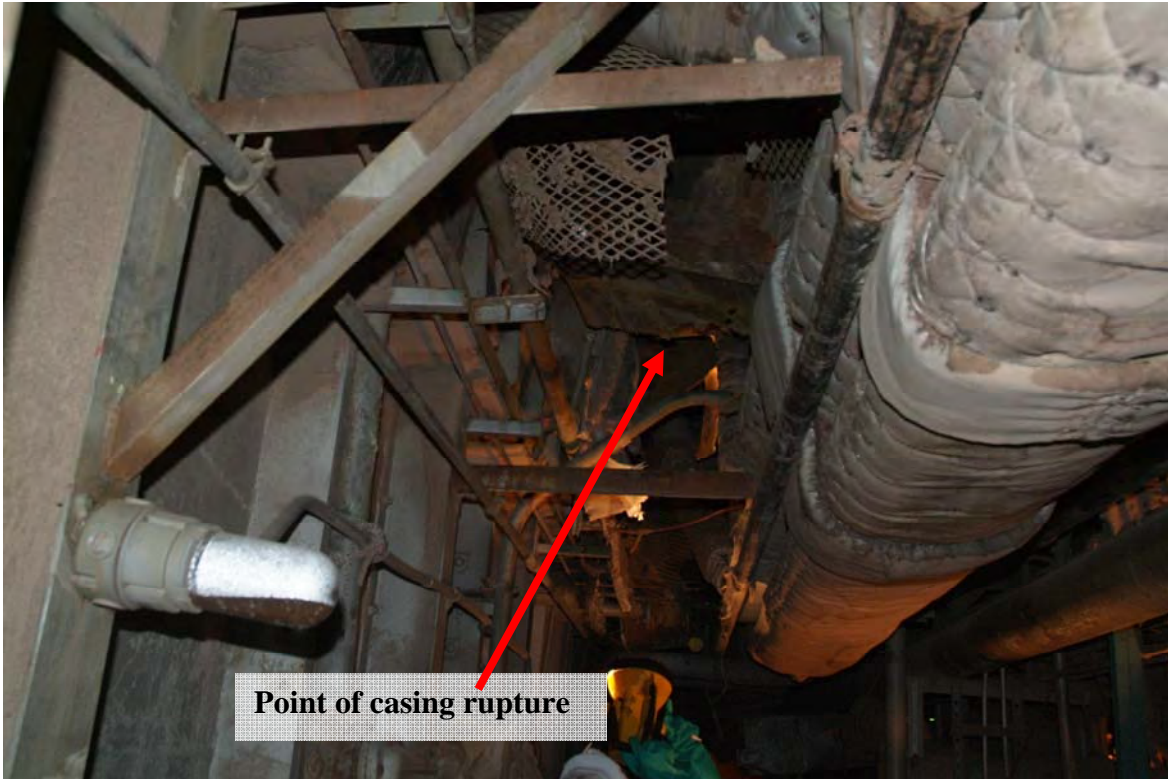
8. Area immediately below casing failure (facing south)
