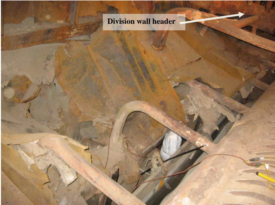
5. Dead air space showing ruptured boiler casing (looking down, facing south)
