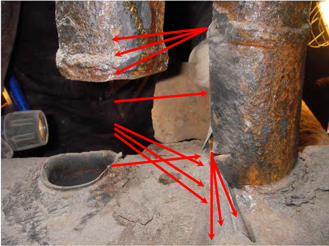
15. Steam impingement indications between tube 9 and 11
