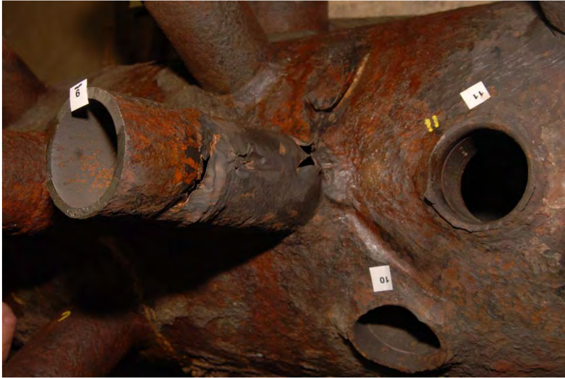
19. Overview of header at point of failures
