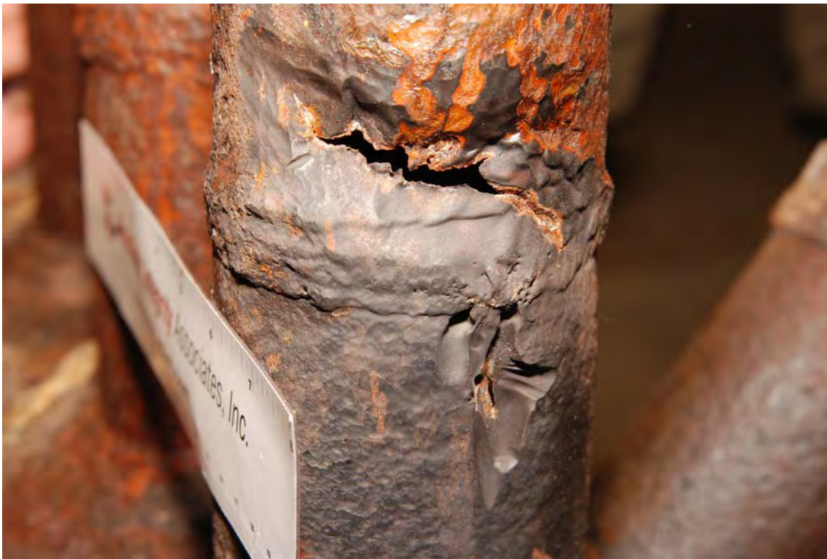
22. Close-up of tube 9 top leaks
