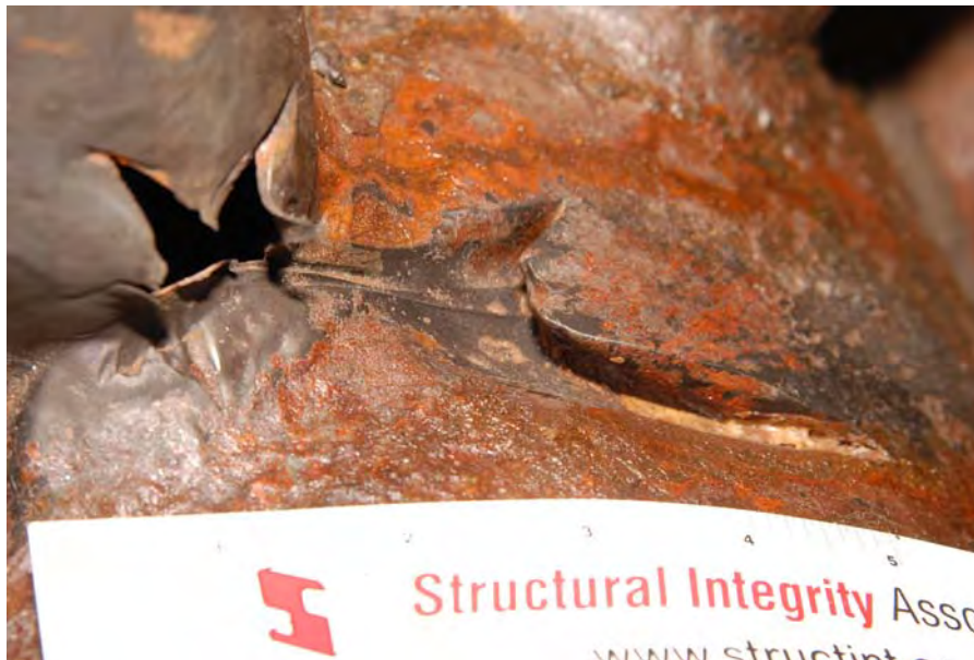
29. Close-up of header damage from steam/water impingement
