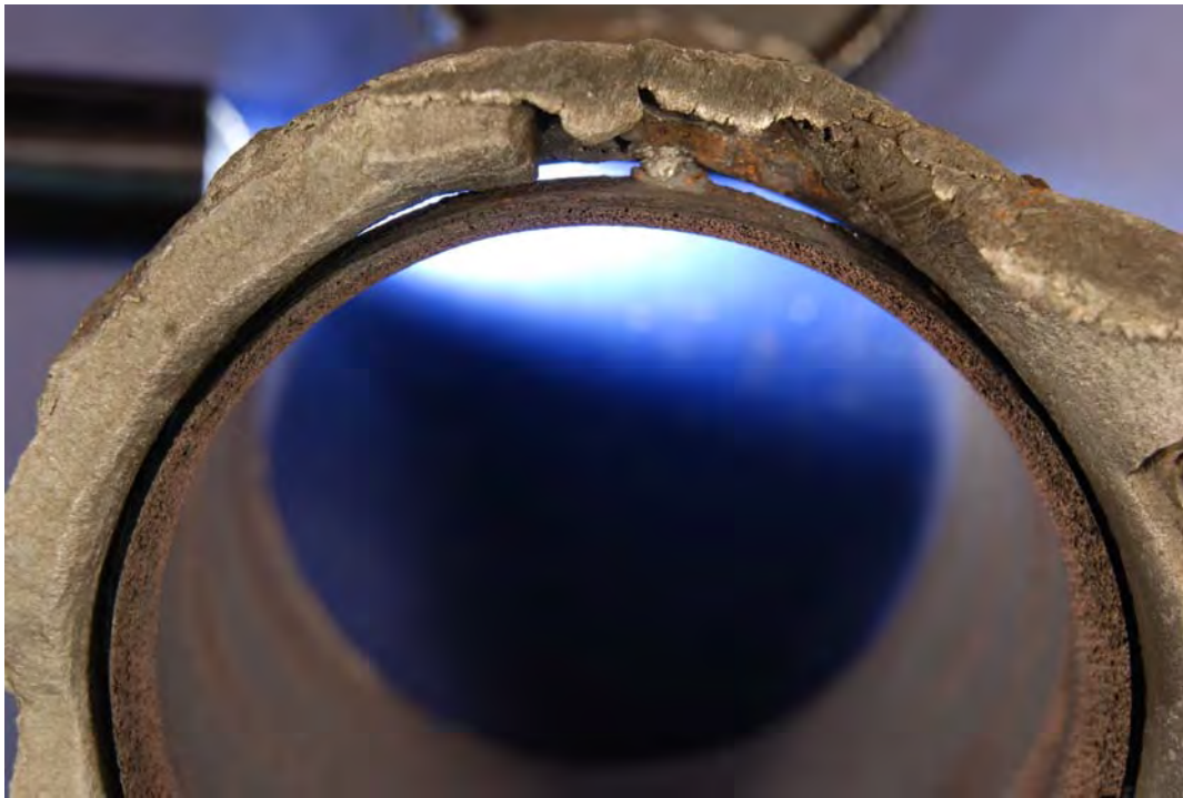
31. Close-up of Tube 10 showing poor weld
