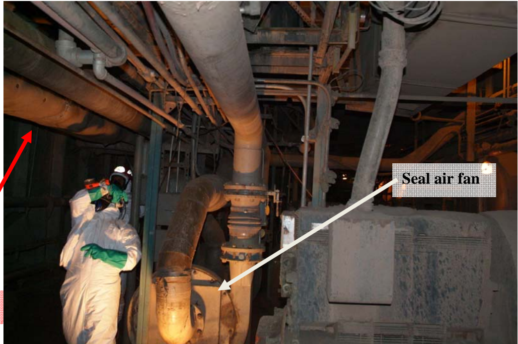
7. Area adjacent to point area below failure (facing south)
