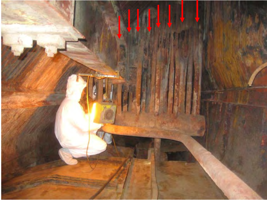
50. West side dead air space after ash is removed. Prior level of ash is evident on division wall header
