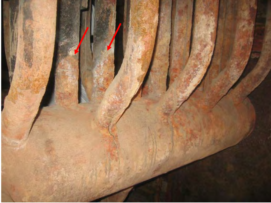
52. West side dead air space after ash is initially vacuumed out. Difference in corrosion in tubes closest to header
