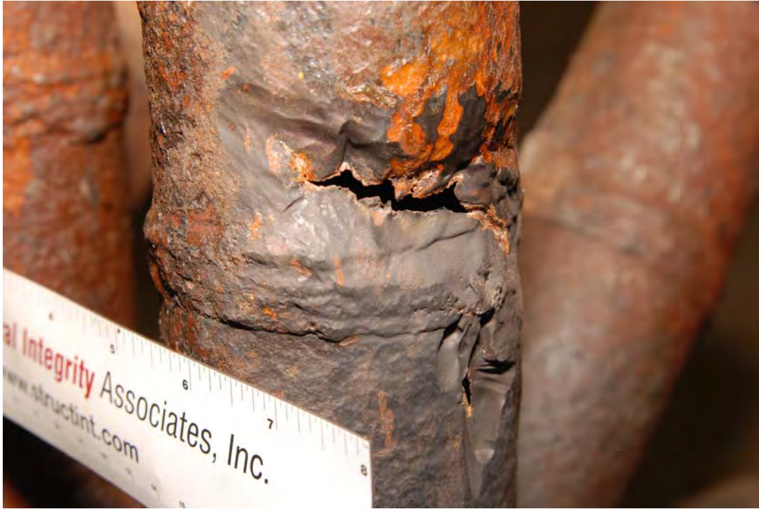
21. Close-up of tube 9 top leak
