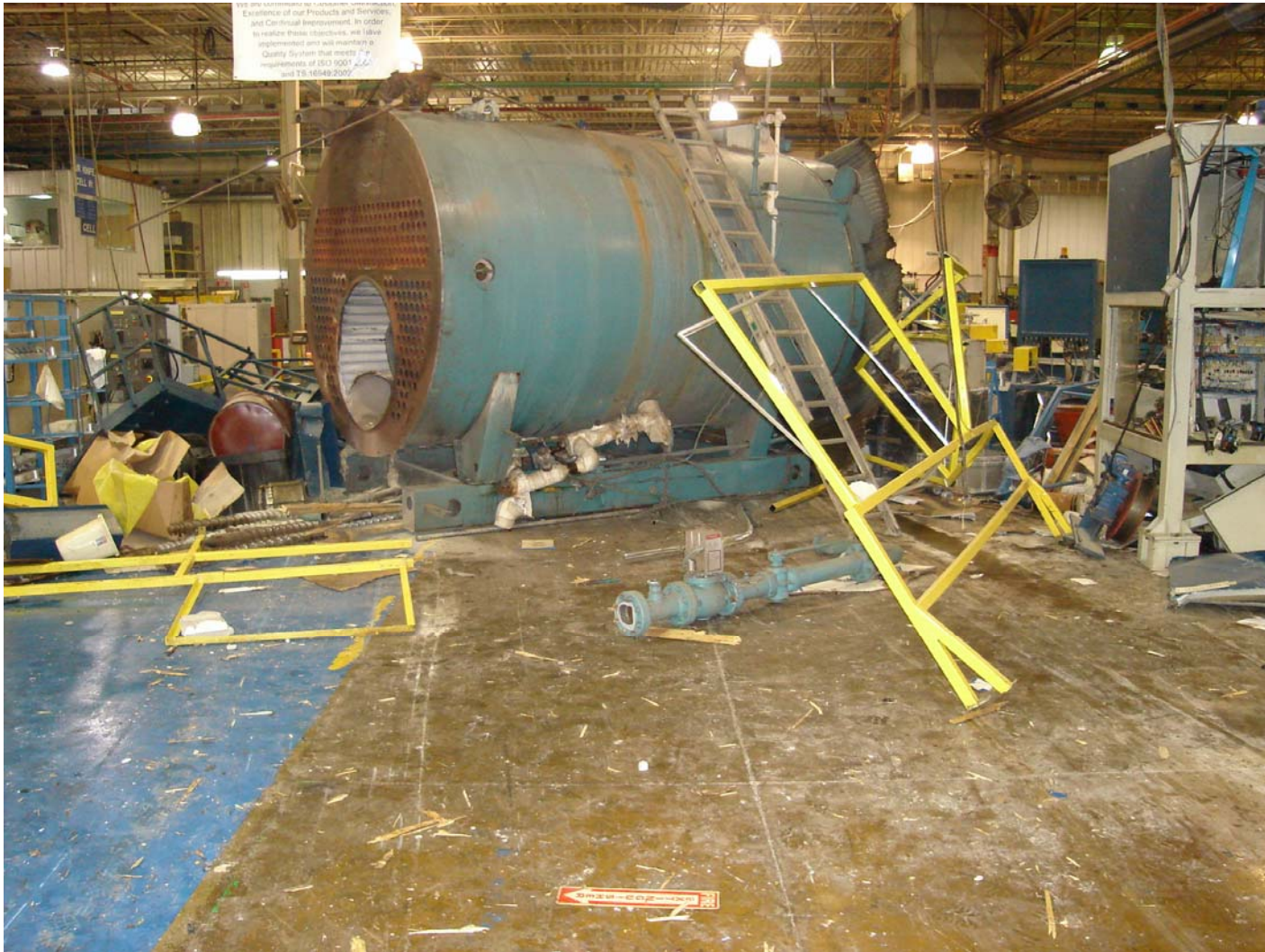
Photo #2 – Final Location of Boiler After Explosion
