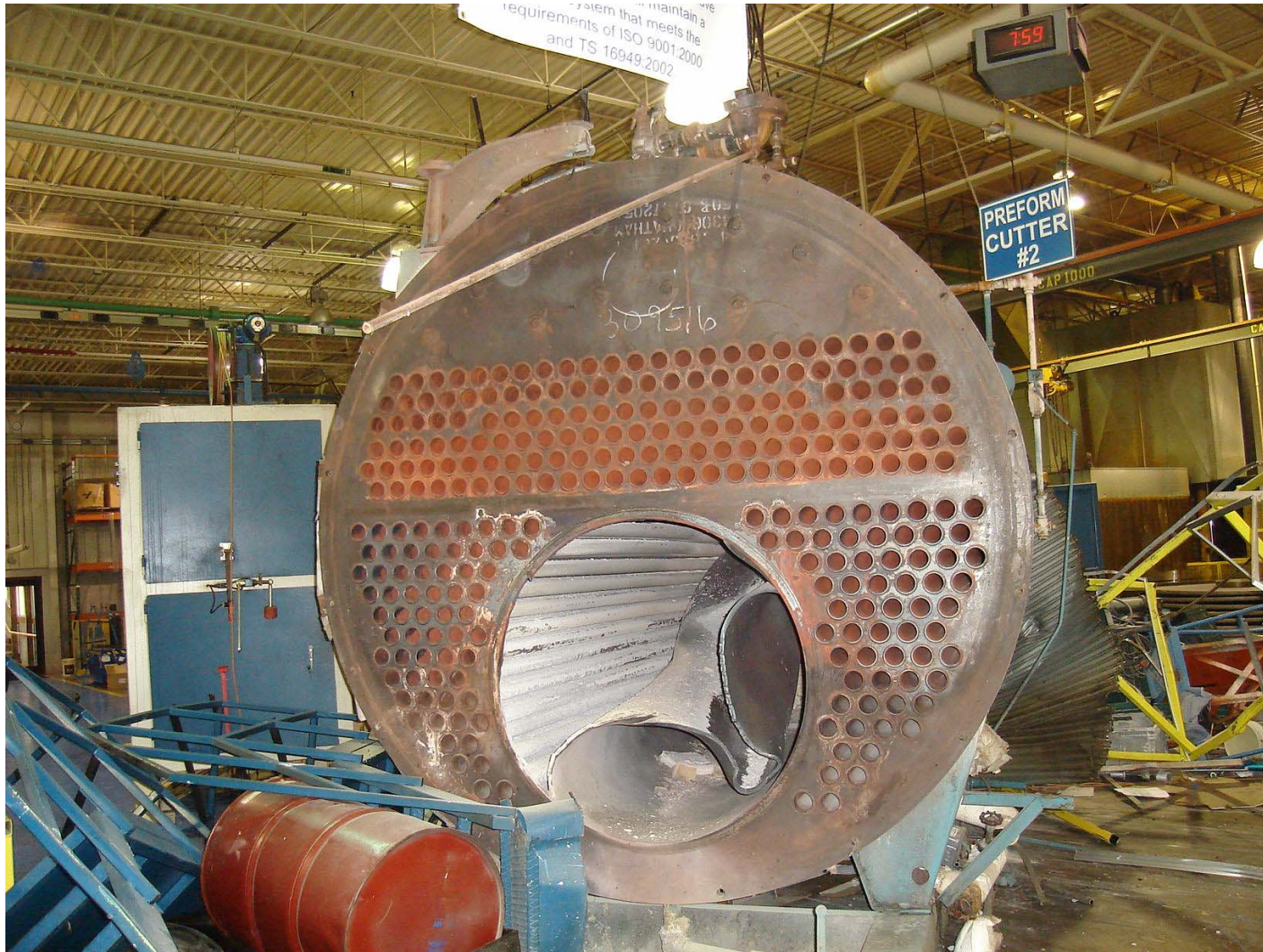
Photo #3 – Final Location of Boiler after Explosion (Exposed Furnace Tube)
