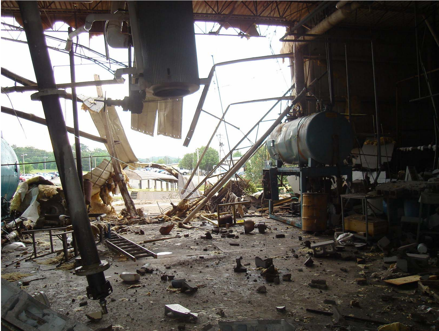
Photo #5 – Knocked Down Exterior Wall Viewed from Inside Boiler Room (East Wall)
