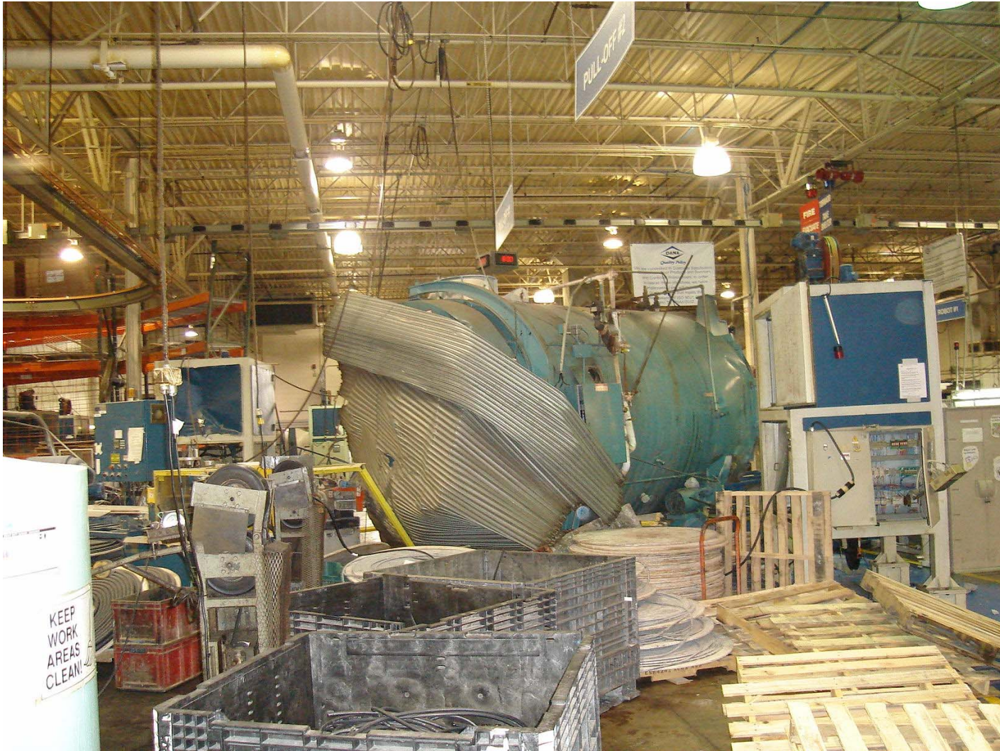
Photo #1 – Final Location of Boiler after Explosion (Roll Up Door on Boiler)
