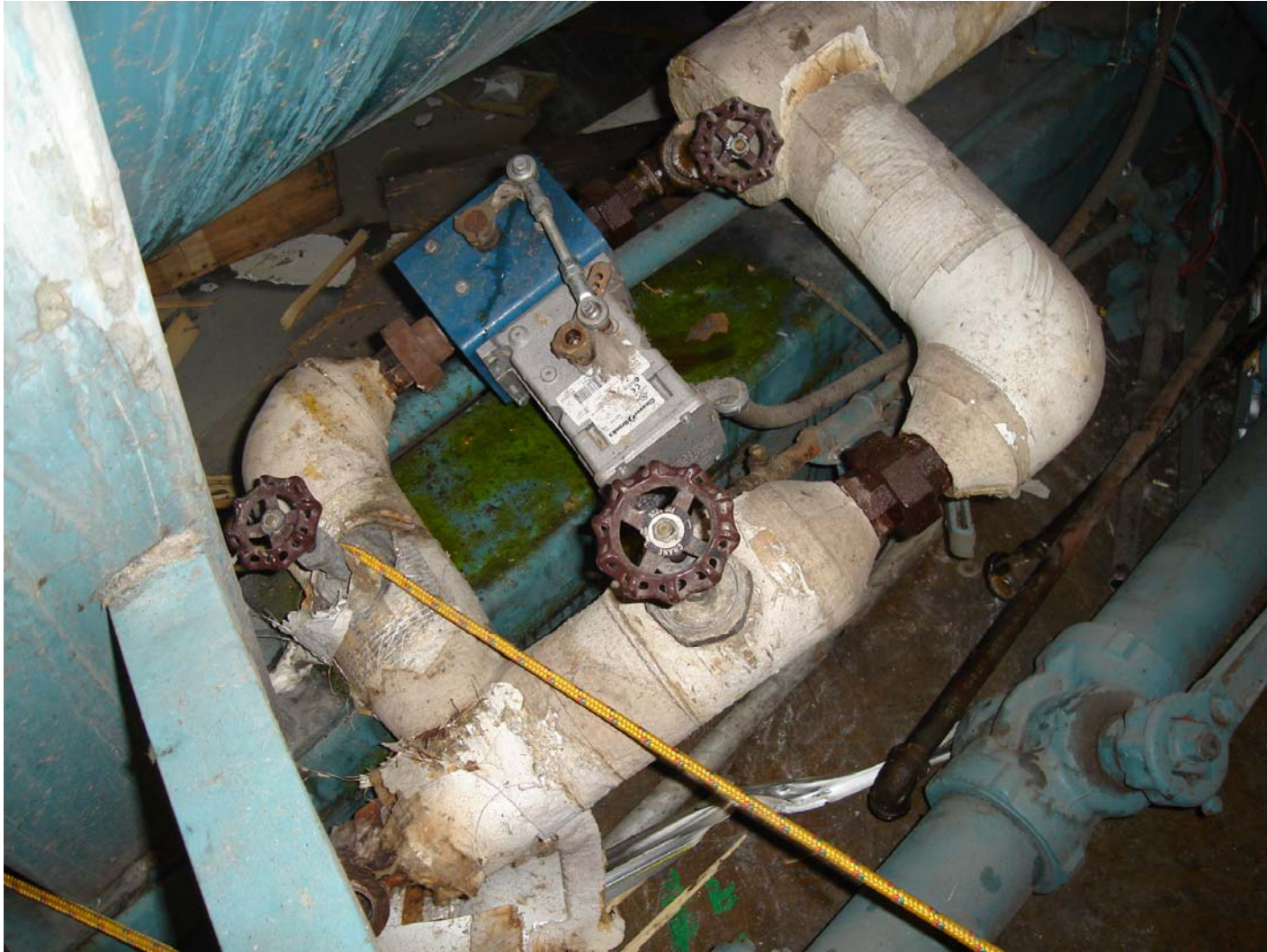
Photo #10 – Modulating Feed Controller, Valve, and Bypass (Note Disconnected Operating Arm)
