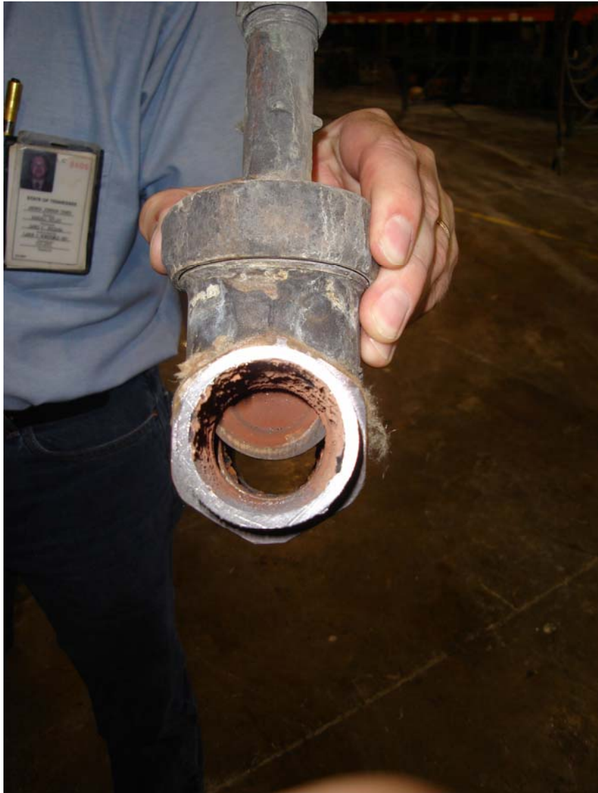
Photo #12 - Bypass to the Modulating Feed Valve. Valve was found in the half open position.
