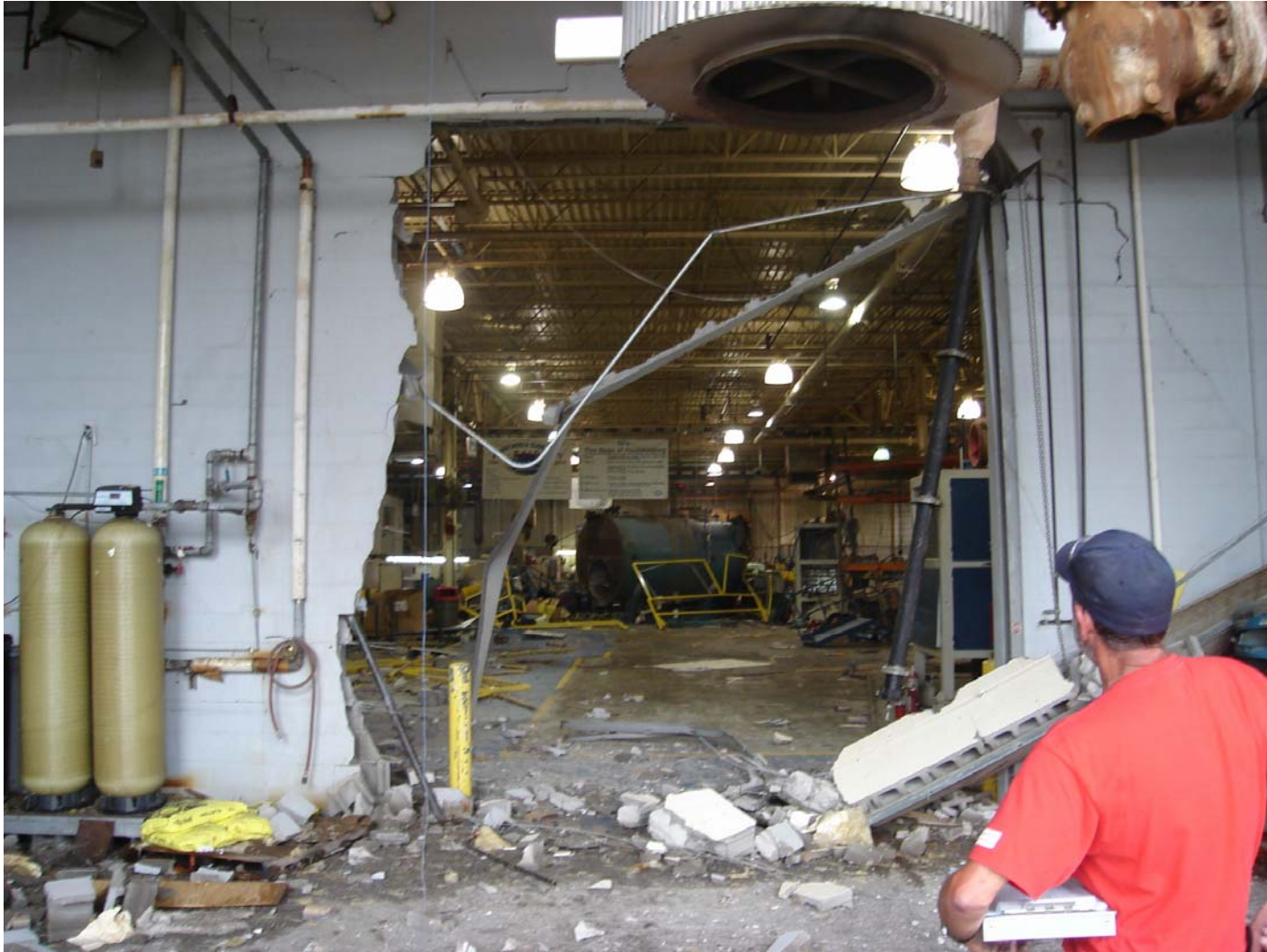
Photo #4 – Hole Created by Boiler through Roll Up Door Wall (West Wall)
