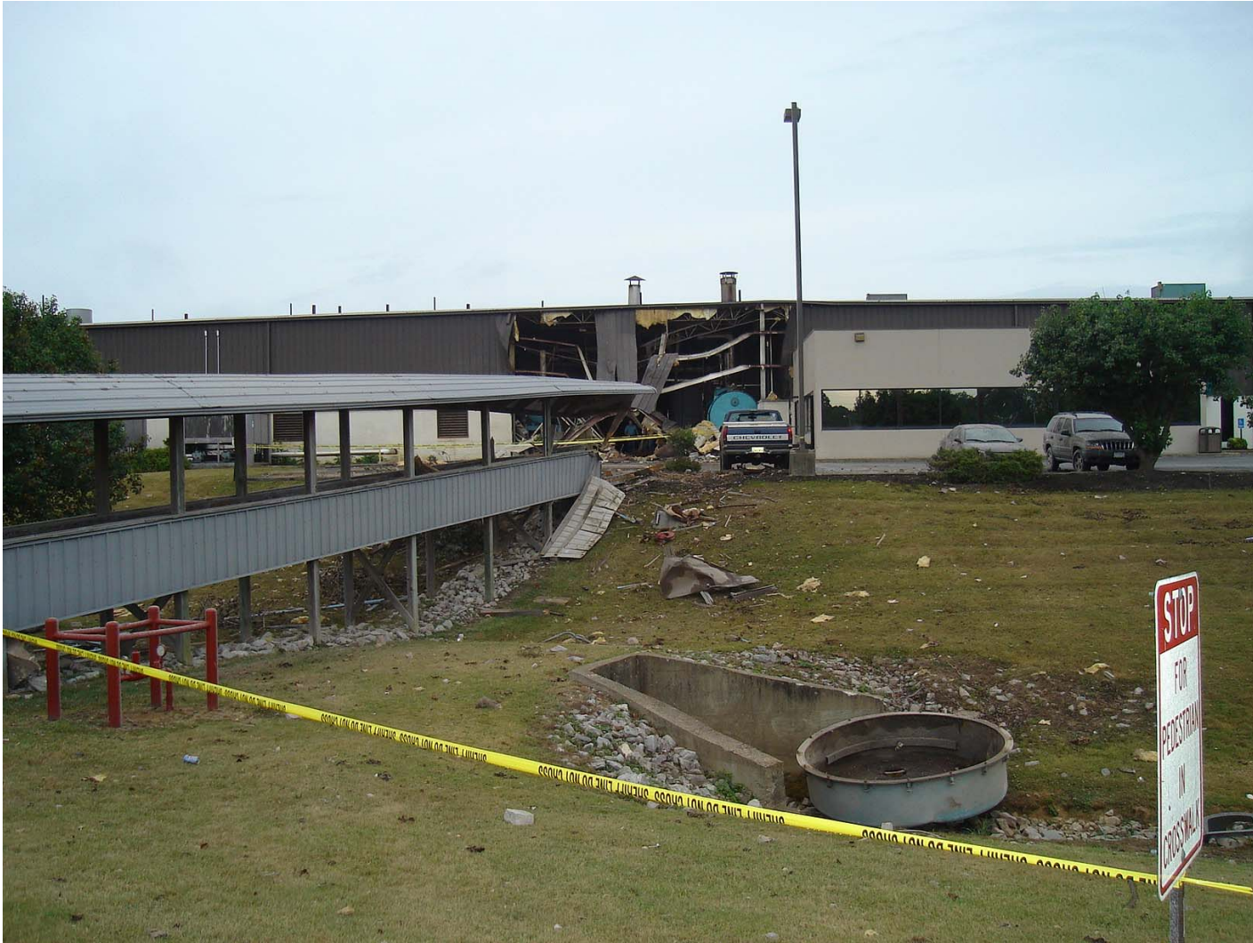
Photo #7 – View of East Wall from Outside Plant (Note Rear Boiler Door in Ditch)
